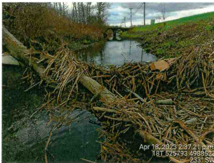
Photo 4: Station 1 looking at the partial woody blockage at its upstream end (April 18, 2023)
