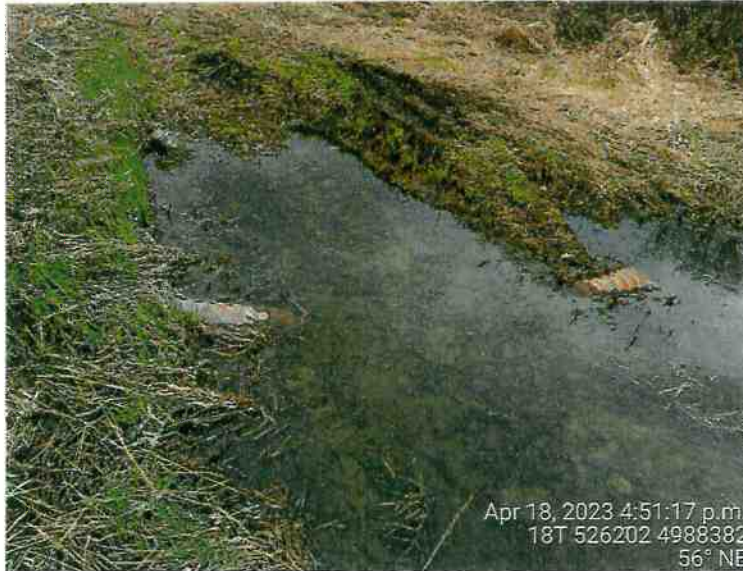
Photo 7: Broken culvert at the road crossing (April 18, 2023)
